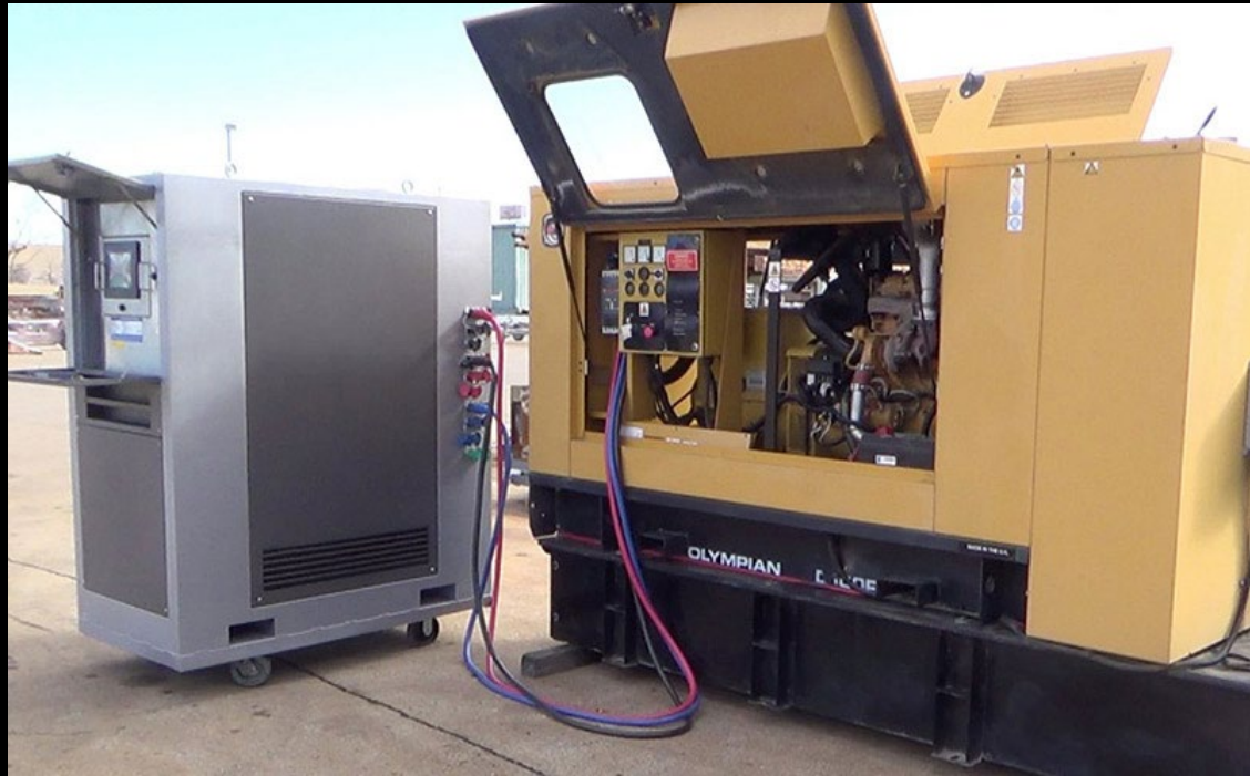
Loadbanks (Permanent or Temporary)
